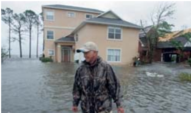
Hurricane Dennis: Dennis caused flood damage to this house in Navarre, Florida, only five weeks after repairs from the previous year's Hurricane Ivan were finished.
