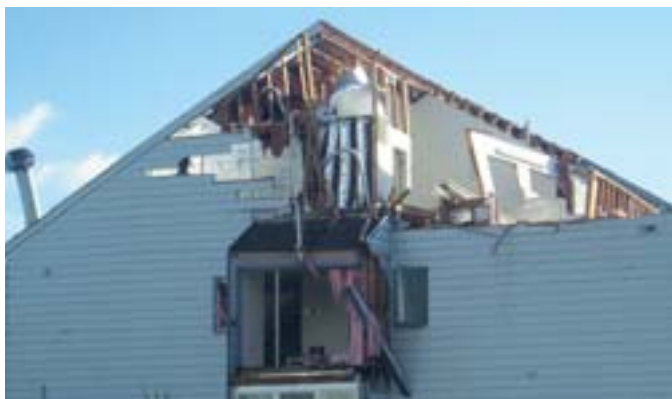
Hurricane Charley: The roofs of dwellings were often torn off, sometimes completely, as in this case in Punta Gorda on the west coast of Florida. This also leads to the contents being severely damaged.
