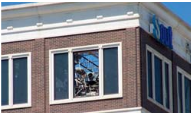
Hurricane Ivan: This office building in Pensacola, Florida, still looks good, but it lost part of its roof during the storm. Older office buildings in the city centres were often badly damaged.
