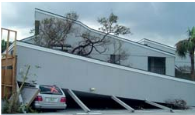
Hurricane Frances: This carport in Florida was not strong enough to withstand the wind pressure of the hurricane.
