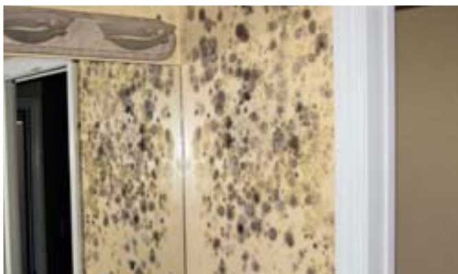
Hurricane Ivan: Mould growth in a hotel on Grand Cayman is promoted by infiltrating moisture and the prolonged stoppage of air-conditioning systems. The power supply had collapsed after Ivan.
