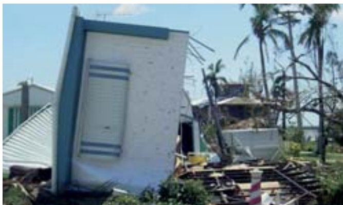
Hurricane Charley: This mobile home in Pine Island put up little resistance to the high wind speeds. Mobile homes contributed significantly to hurricane losses in 2004.
